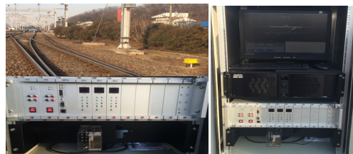
Fig. 10. ACS interfaced with Interlocking System at Cheong-Ju station
