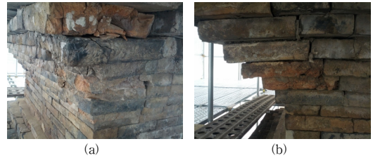
[Fig. 13] Damage and spacing between member (Andong Jotap-ri 5-story brick pagoda Conference Material Reference) (a)Damage (b)spacing
