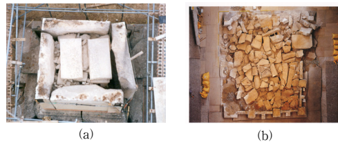
[Fig. 4] stone pagoda Jeoksim(Jang Suk-Ha, Chung Hae-Doo, A study on characteristics of composition method of inner foundation in stone stupa Reference) (a) Nawon-ri (b) Mireuksa
