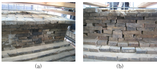
[Fig. 12] Separation and damaged separation between members(Andong Jotap-ri 5-story brick pagoda Conference Material Reference) (a) Separation phenomenon (b) Damage separation phenomenon
