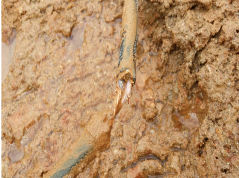
Fig. 12. Half open fault of cable
