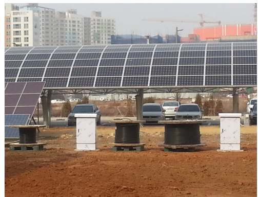
Fig. 15. Outside distribution board and cable for distance extension
