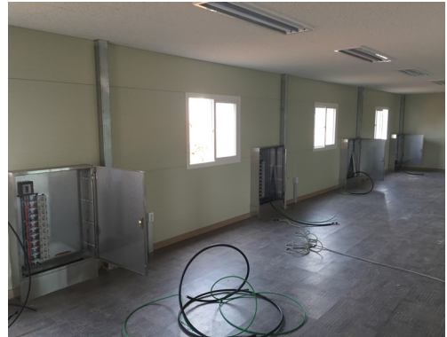
Fig. 13. Inside distribution board for installation of cable fault locator in the cable test building
