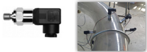
Fig. 8. Pressure sensor and installation on the pipe
