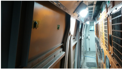
Fig. 9. Temperature sensor attached surface
