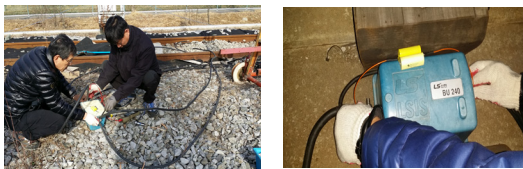
Fig. 14. 6m Cable connect Fig.15. Capacitor addition
