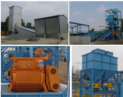
Fig. 1. Twin mixer batch plant
