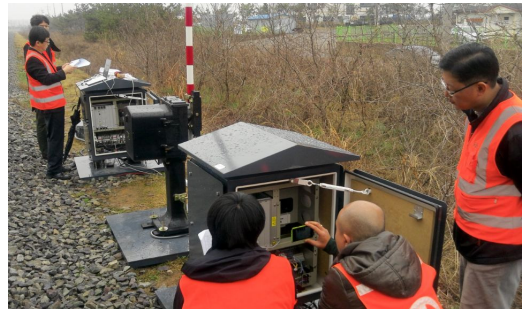
Fig. 5. Crossing gate control via Ethernet
