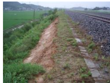
Fig. 2. Slope failure of embankment
