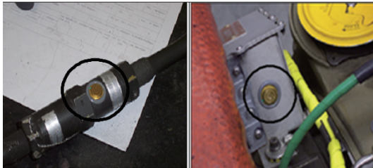
Fig. 1. Attachment Shape of CMB (Oil Pump & Electric Circuit Box)
