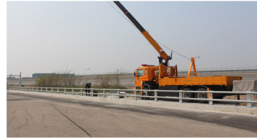
Fig. 7. Installation view of final modified bridge barrier for the actual crash test
