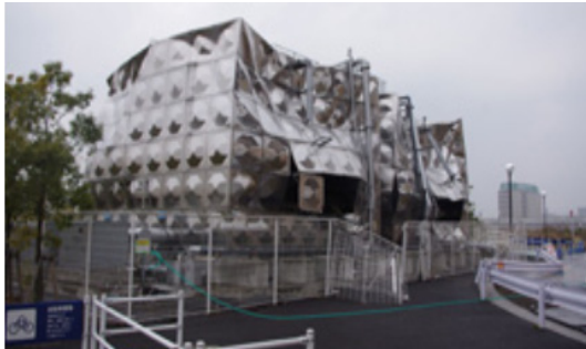
Fig. 1. Damage to Large Stainless Steel Panel Tank (Natori City, Miyagi Prefecture)
