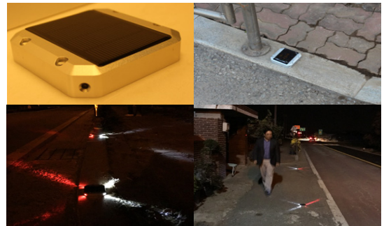
Fig. 9. Recognition light on the road for the underprivileged in traffic installation view
