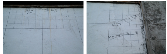
Fig. 15. Cracks on shrinkage restricted concrete wall without w/o using shrinkage reducing agent
