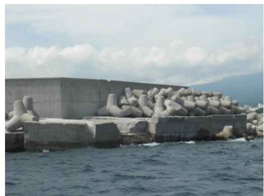
Fig. 2. Damage of breakwater in Seogwipo port, Jeju
