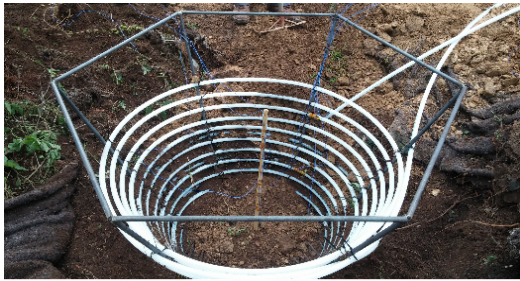
Fig. 3. Geothermal heat dump
