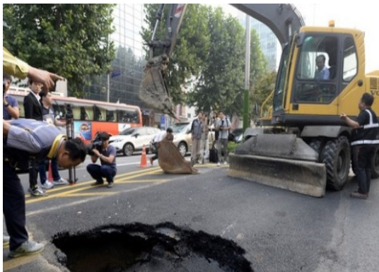
Fig. 2. Road subsidence caused by pipe damages
