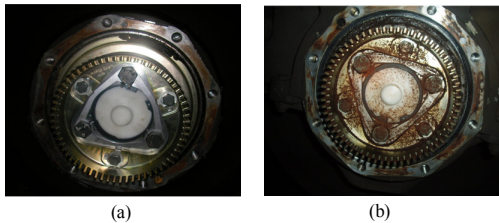
Fig. 4. Bearing condition on 7th(a) and 8th(b)
