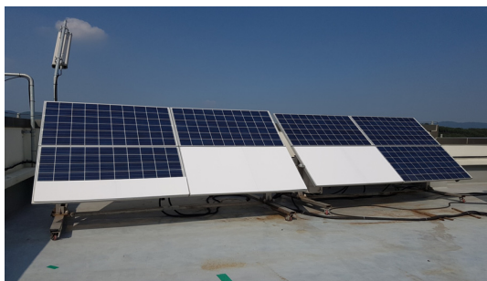
Fig. 10. Shading Experiment condition of the Photovoltaic modules
