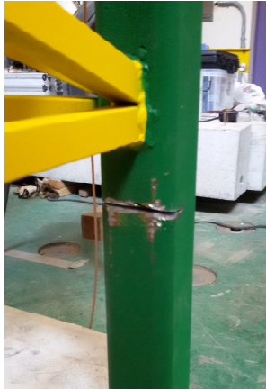
Fig. 9. Inflicted damage (Case 2)
