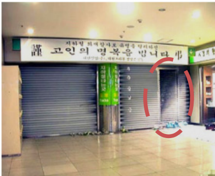
Fig. 1. Daegu Subway Iron Fire Shutter('03)
