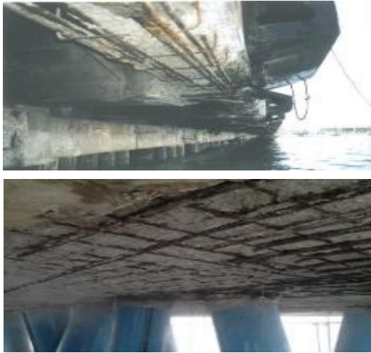
Fig. 1. The Illustrations of Harbor Structures Concrete Deterioration
