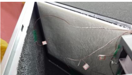
Fig. 11. A photo of freezing in case of -20^{\circ}\text{C} of OA temperature and 22^{\circ} open of recirculation damper.
