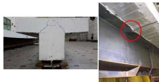
(b) Cracks of end section
