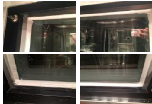
Fig. 13. Appearance of specimen after 400cycles (Modified Silicone Sealant)
