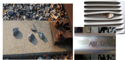
Fig. 1. Damage of track facilities due to scattering of railway ballast on the sleepers
