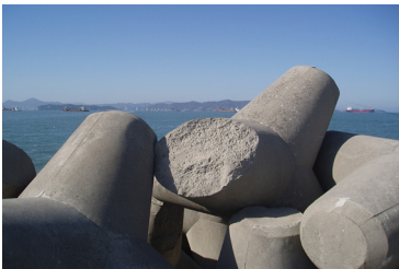
Fig. 2. Partial damage of concrete block on the ground
