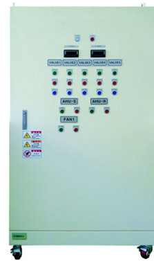
Fig. 6. Control panel of gastight shutdown valve
