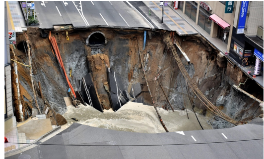
Fig. 1. Subsidence and sink hole in road
