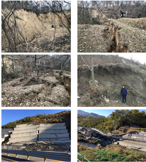
Fig. 1. Photograph of the slow-moving landslide damaged area
