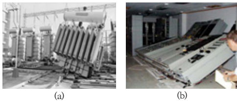
Fig. 1. Earthquake damage case (a) Sichuan earthquake damage case (b) Taiwan earthquake damage case
