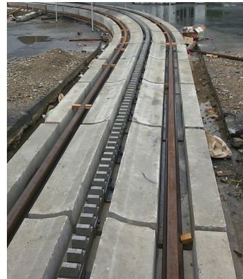
Fig. 2. Concrete embedded rack track
