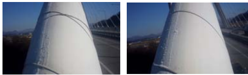
Fig. 6. The condition of cable surface after operating snow removing robot
