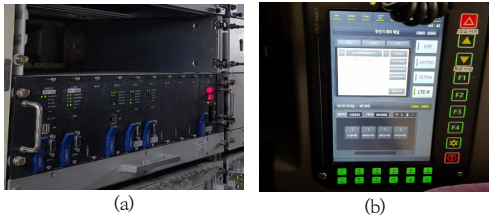
Fig. 2. On board units of LTE-R (a) TCI (b) TRCP
