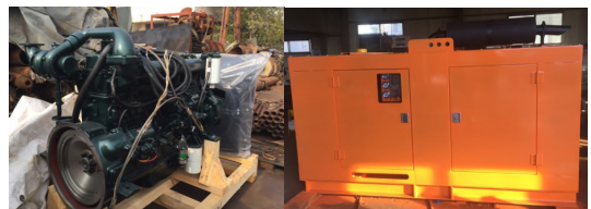
Fig. 4. Engine and power pack system
