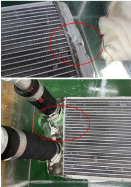
Fig. 8. Leakage point of existing heater core
