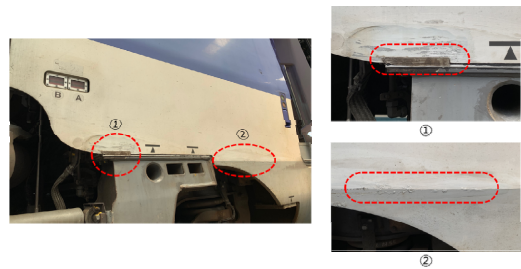
Fig. 8. Inspection zones ① and ② for connection weld between carbody and bogie
