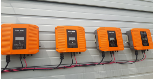
Fig. 5. Solar inverter's place
