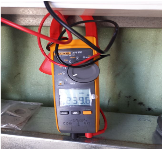
Fig. 6. Voltage after Inverter 3 on
