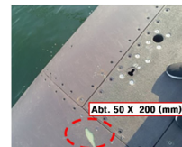
Fig. 8. Delamination of the gel coat during the test.
