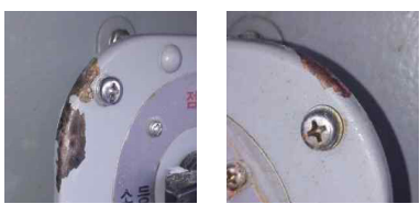
Fig. 3. Corrosion on rotary switch
