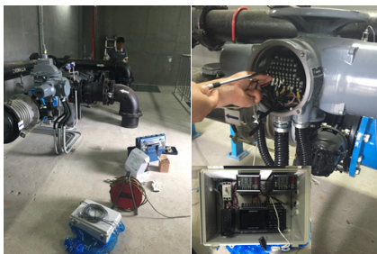
Fig. 11. Experimental testing for water hammer control
