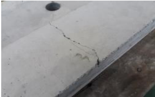
Fig. 7. Crack on precast concrete
