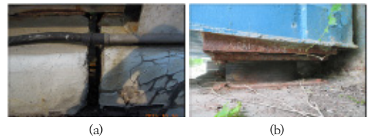
Fig. 4. Damaged components of bridges due to damaged expansion joints (a) Deck (b) Bearing Rust
