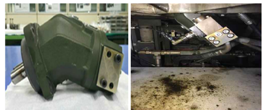
Fig. 1. Hydraulic fan motor and oil leakage
