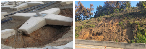
Fig. 2. Slope surface failure and erosion
