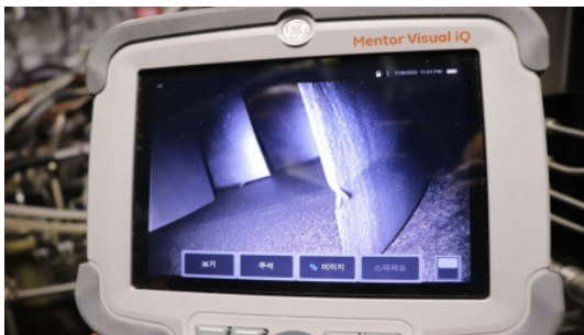
Fig. 2. Compressor of gas turbine on stage #1 through borescope
