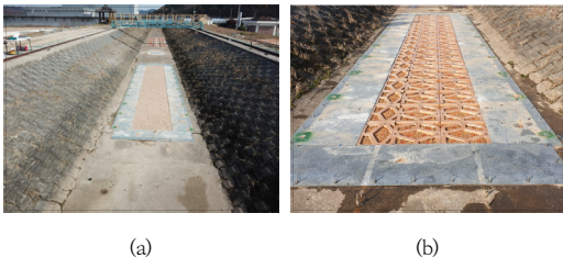
Fig. 4. Installation of biodegradable block for experiments(no vegetation) (a) front view, (b) plan view
