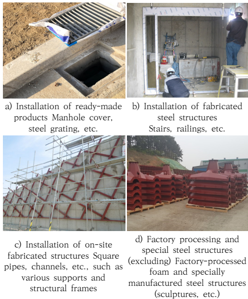
Fig. 2. Example of type of production installation
