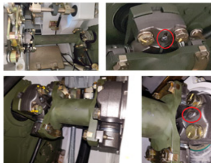
Fig. 14. System installation test result
