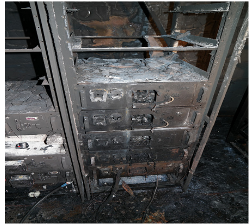
Fig. 12. Checking battery condition after complete fire extinguishing in top fire stage of 25kWh Rack
