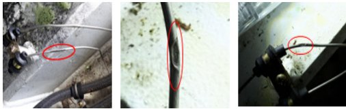
Fig. 3. Damage to Fire Detection Wire
